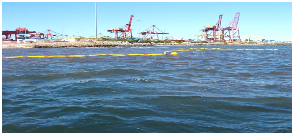
Photo: 4 – Photos 2, 3 and 4 demonstrate silt curtains failing only a few days after works have begun.
